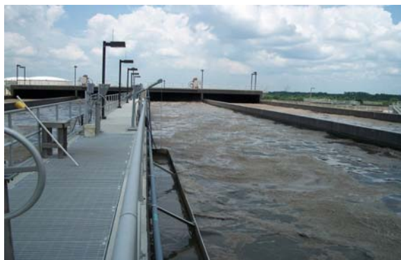
Prior to installing ChemScan online process analyzers, operators manually adjusted blower speed at the control boxes located near the aeration basins.
